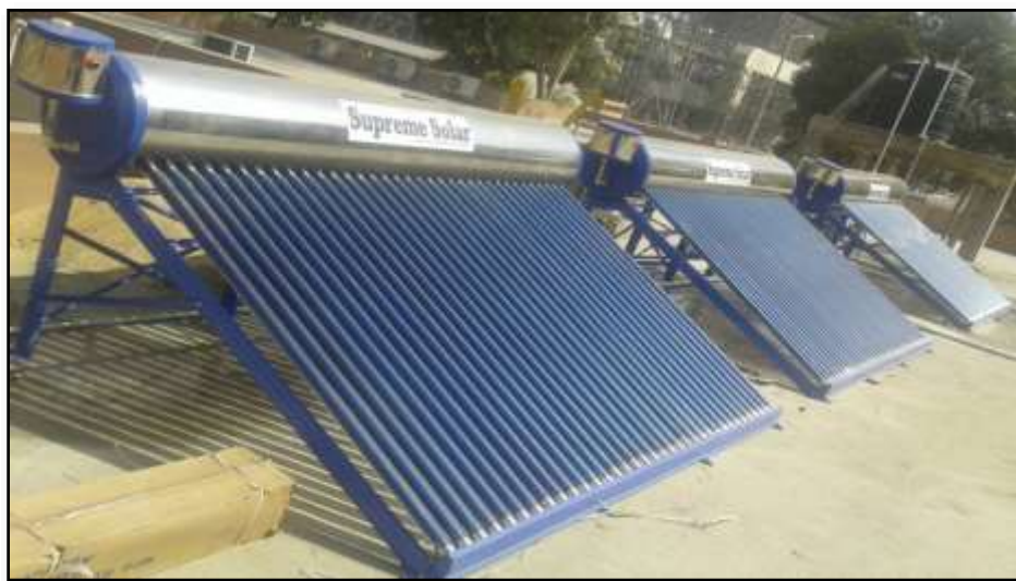
Solar Water Heater at Plant
