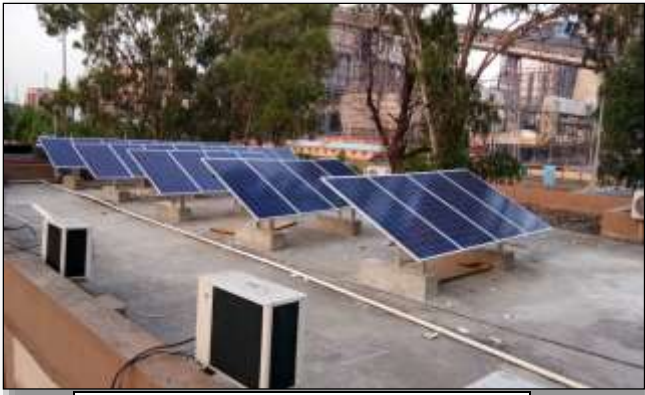
Solar PV Plant in Canteen.
