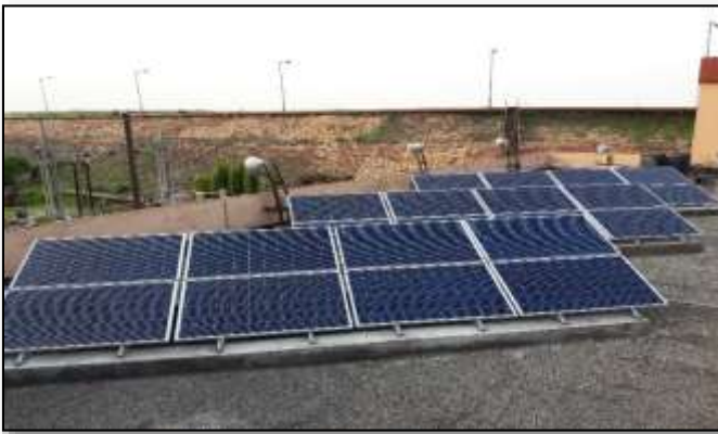
Solar PV Plant in Ash Pond.
