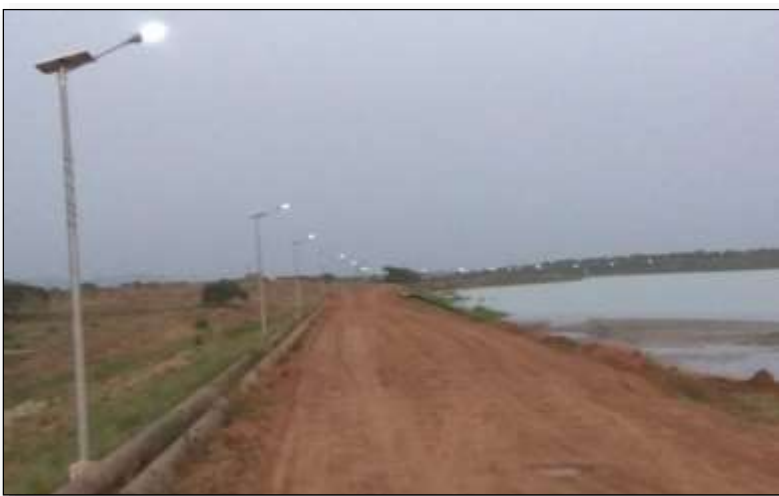
Solar Powered LED Street Light at Ash pond-C
